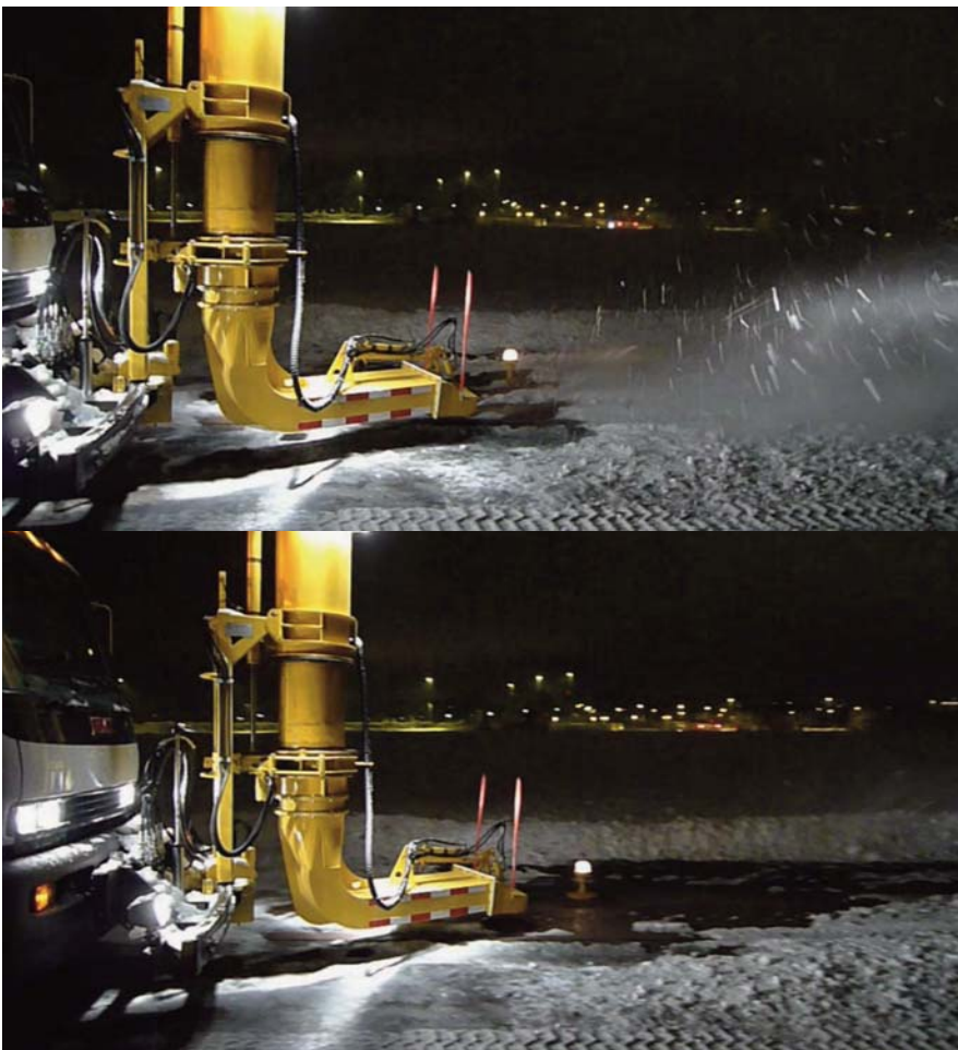
The AF1 cold air blower cleaning runway lights.
